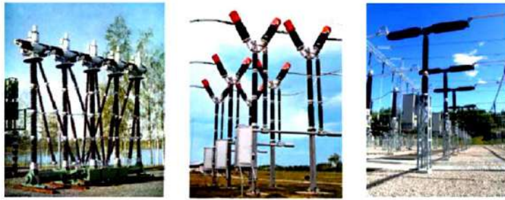
Air Blast Oil Minimum SF 6 Gas
